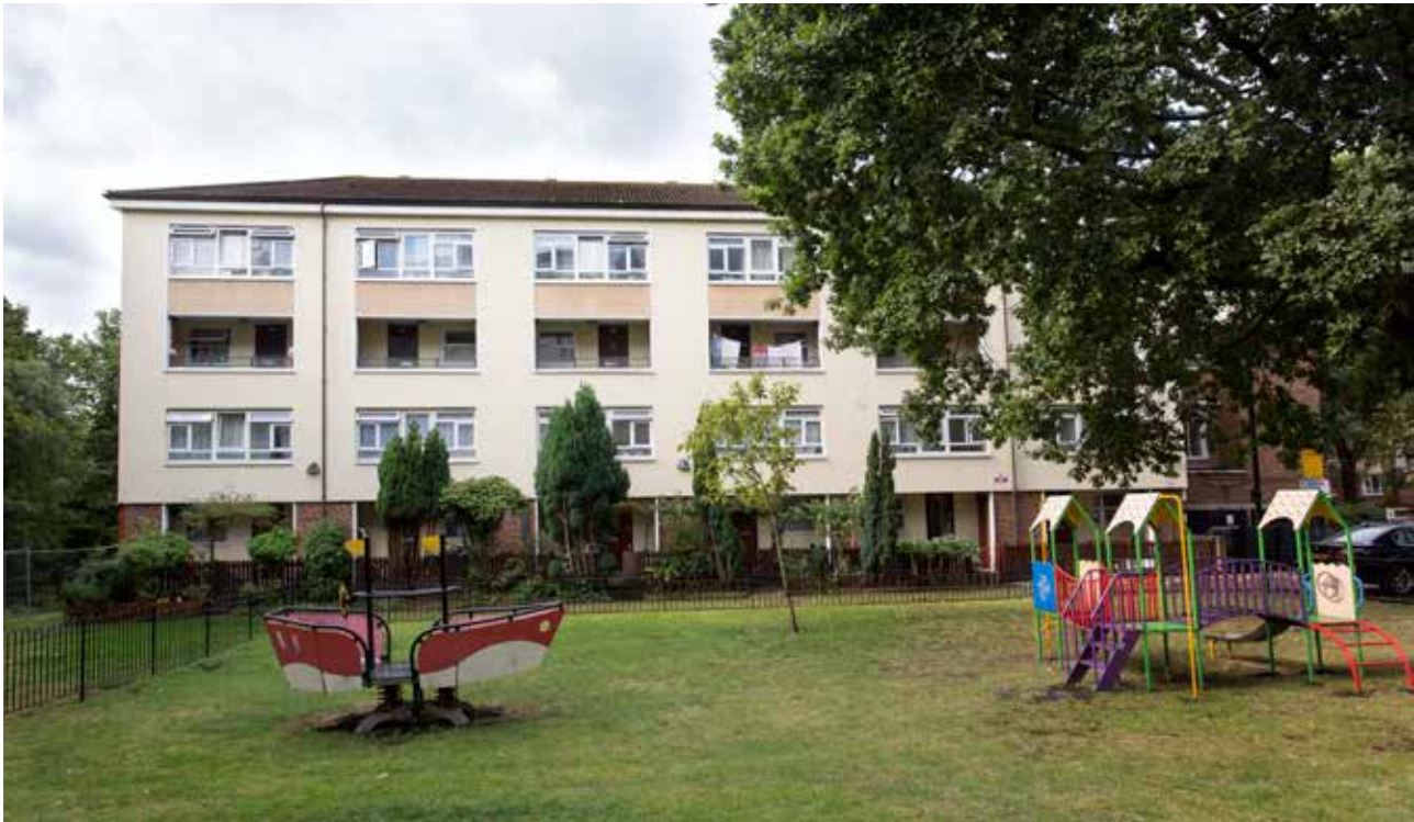
Figure 16. External wall insulation has been installed on blocks in the Holly Park estate
