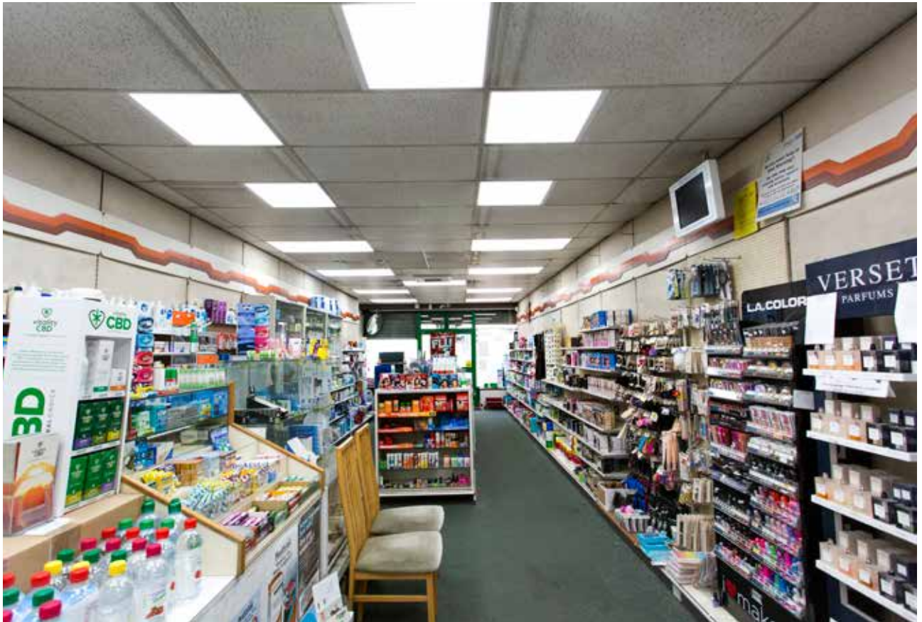
Figure 28. LED lighting installed at a local business through the Energising Small Business fund
